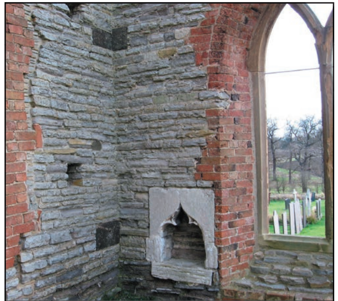
Figure 3. Southeast corner of the Chancel with Blue Lias rubblestone enclosing a piscina carved from a block of oolite adjacent to a C19th window.
