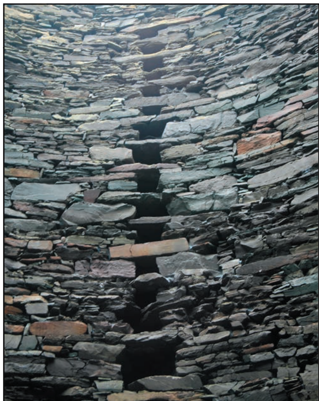
Devonian flagstones used to build an Iron Age broch on the isle of Moussa, off the east coast of southern Mainland.
